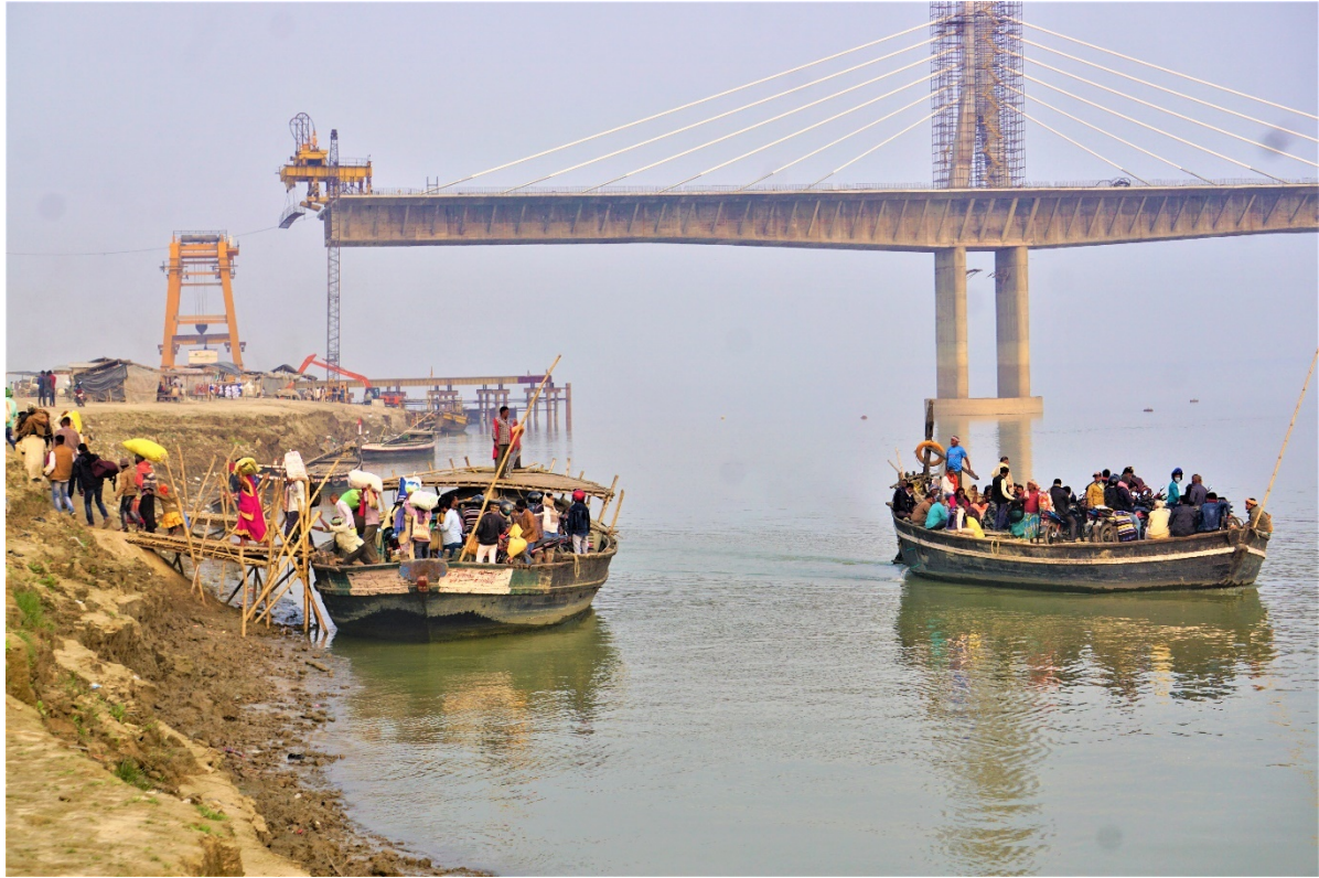
Image 44 : Ferrying At Aguwani Ghat [Bridge over Ganga River is under-construction. It will connect the flood affected North Bihar to South Bihar]
